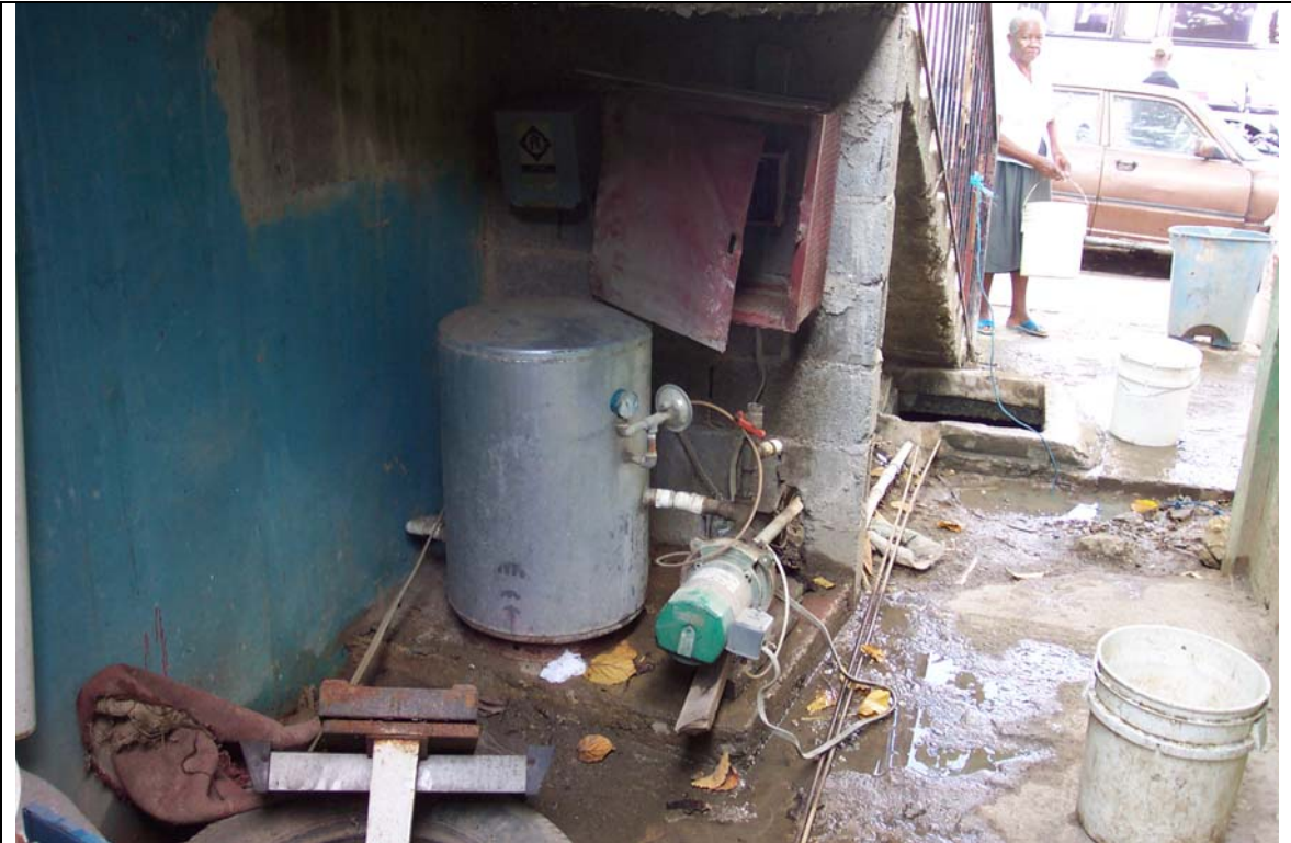
The Jet Pump and Pressure Tank in the Foreground, the Cistern in the Background
